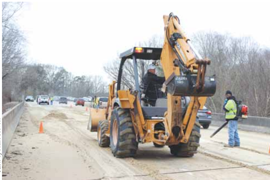
CLEARING SAND from the Comite River Bridge on Hwy. 64. IBTS director David Ratcliff plowed sand off the bridge. The sand was placed there to reduce icing.
