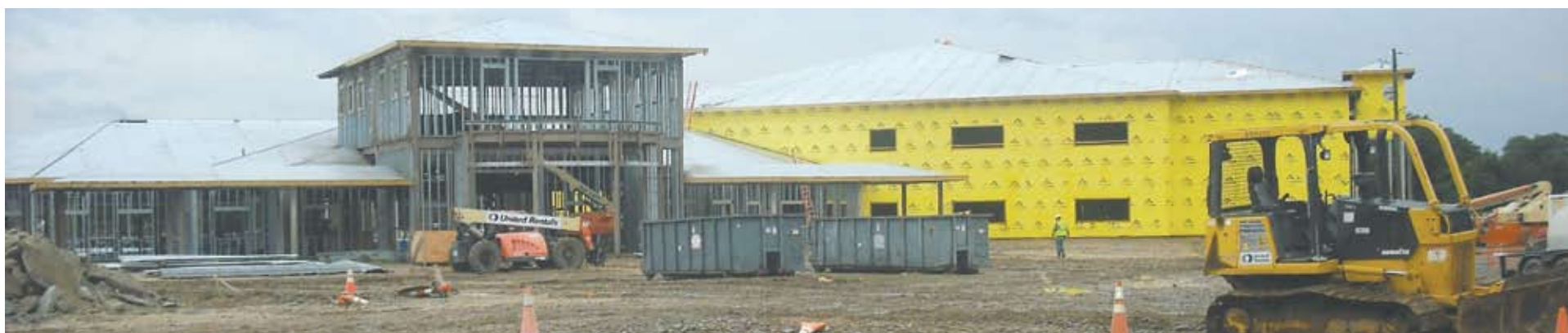
CENTRAL SCHOOL COMPLEX — On Sullivan Road just north of Gurney Road, the new $44 million Central School Complex will include middle and intermediate schools
