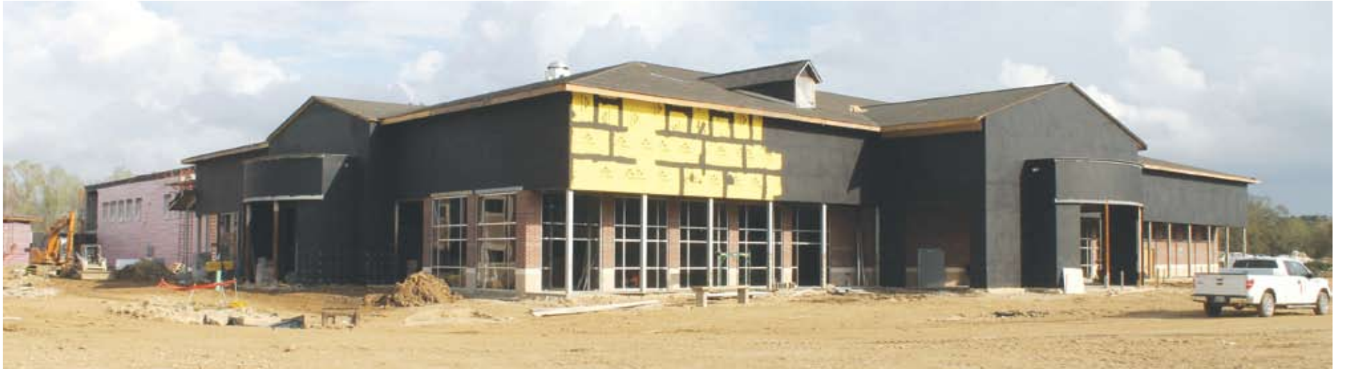
CAFETERIA BUILDING — The cafeteria building at the School Complex will have 32,316 square feet and offer a large dining hall. Outside stages are shown at left and right.
