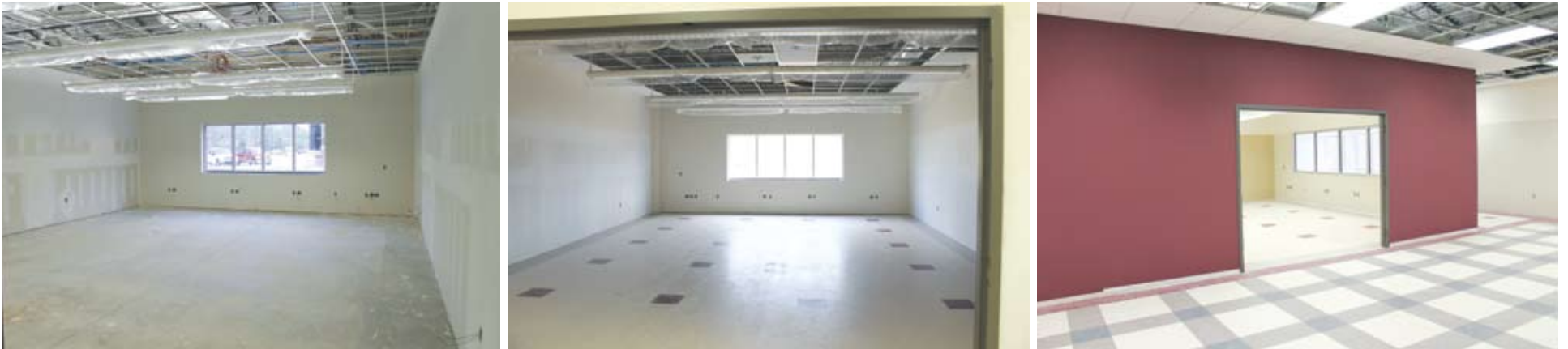
CLASSROOMS IN INTERMEDIATE SCHOOL — Classrooms are also in different stages of completion, ranging from an unfinished shell to nearly complete (left to right).
