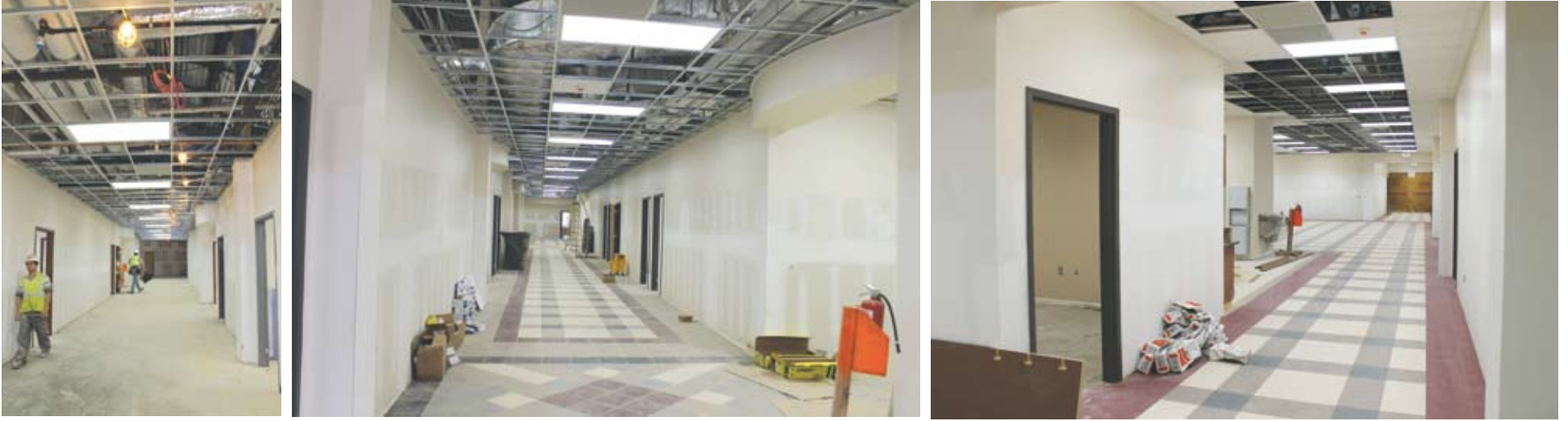
HALLWAYS IN CENTRAL INTERMEDIATE SCHOOL — Hallways in the intermediate school are in various stages of completion. Photos (left to right) show progress.
