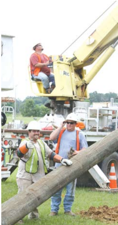
A contract crew from CA-PAR Electric, Inc. installing a pole on Wax Road.
