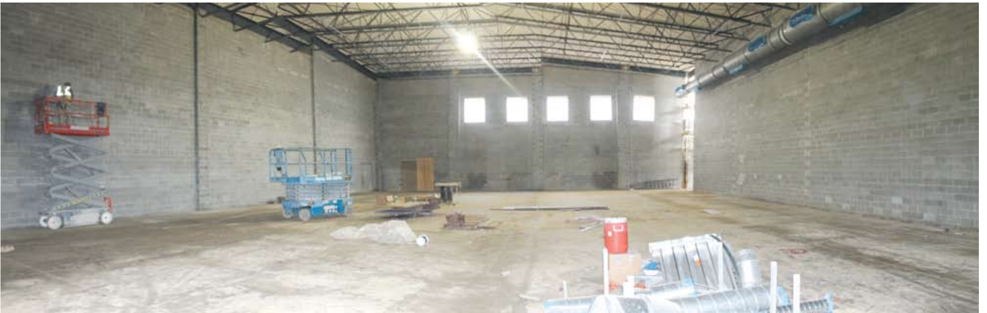
COMPETITION GYM — The competition gym will include a basketball court and can be configured for two volleyball courts. A small set of bleachers will be installed.
